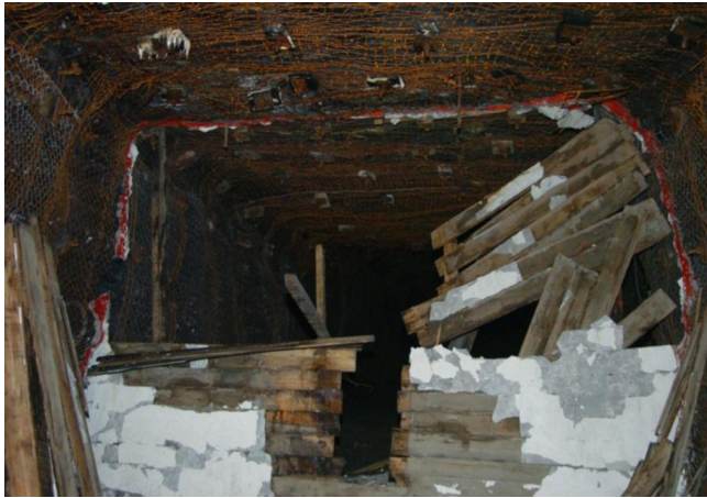
Fig. 2. Airproof wall destroyed by strong tremor happened on 6 September 2004.
