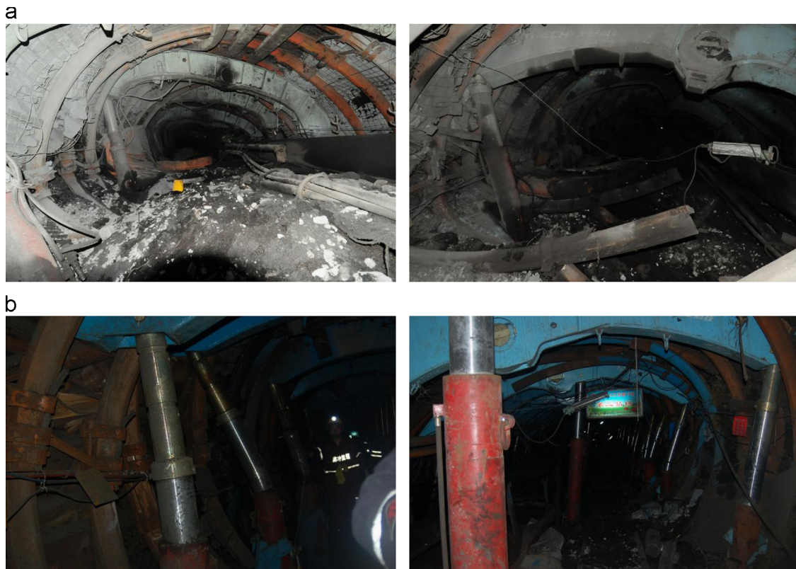
Fig. 10. Photographs of gateway damage taken after rock bursts occurring on (a) 11 August 2010, and (b) 1 March 2011.
