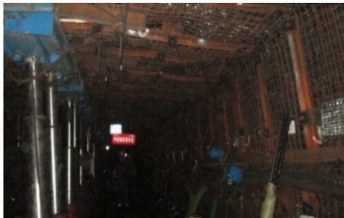
图 12 巷道总体支护效果 Fig.12 Overall support effect of roadway
